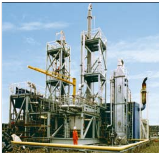
Test plant at Kårstø for removing CO 2 from flue gas. (Courtesy: AkerKvaerner.)
